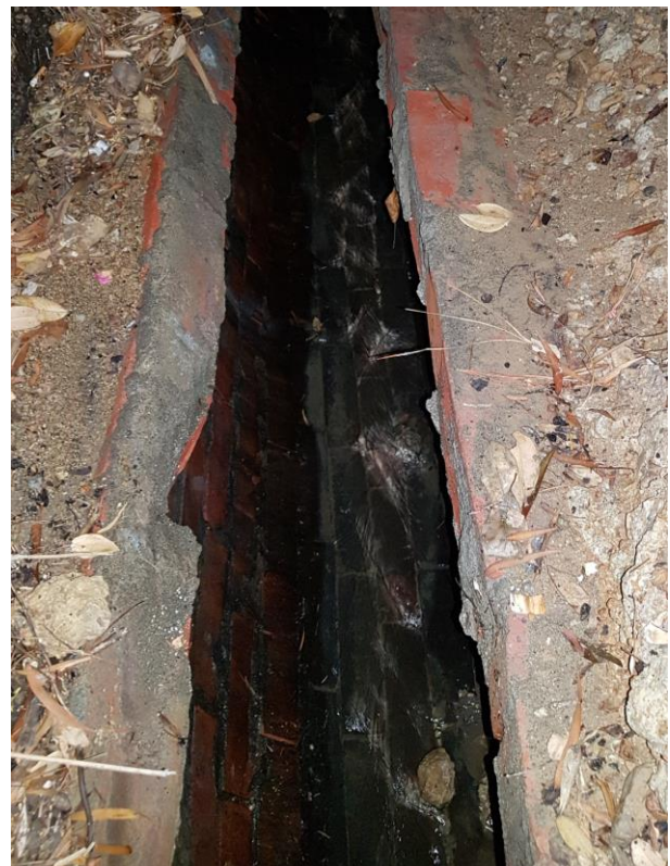
The stormwater surge had blown out the top brick courses of the culvert into the basement of the house
