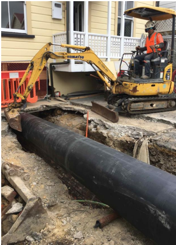
The stormwater surge had blown out the top brick courses of the culvert into the basement of the house
