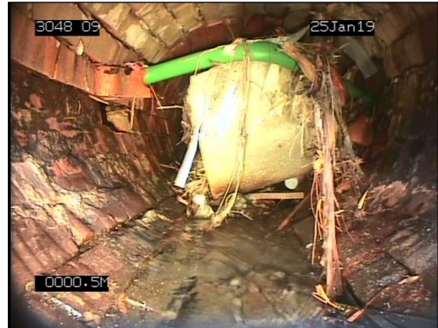
CCTV showing the blockage in the existing culvert
