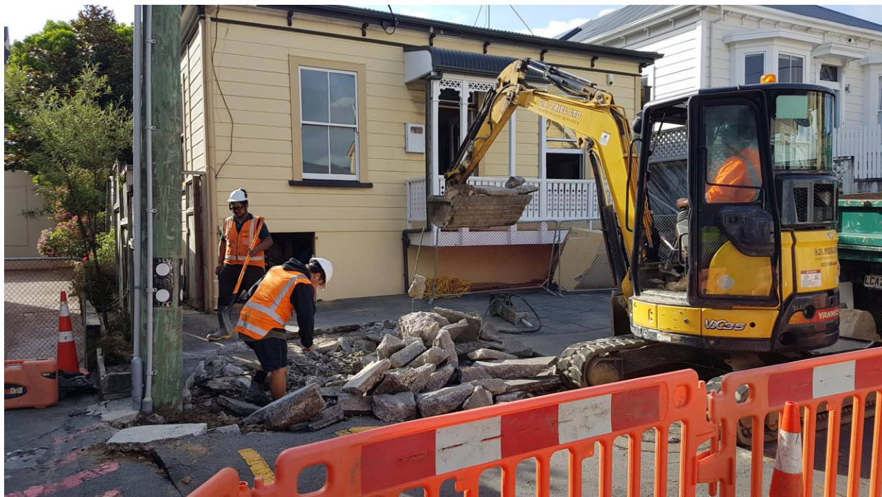
Dan, Lindin & Cody excavating in a driveway to expose the damaged culvert
